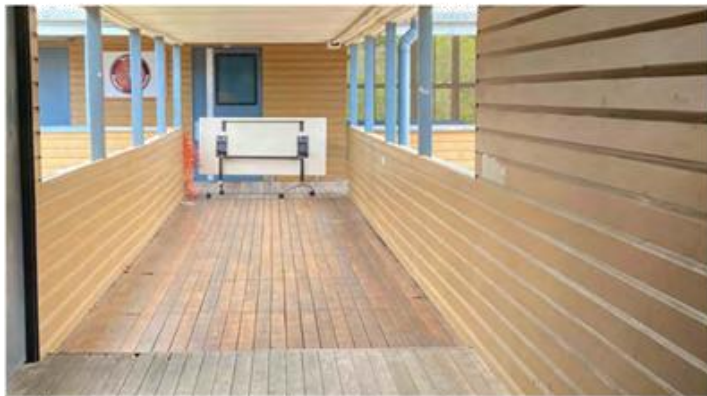
Link block B to block A is condemned
